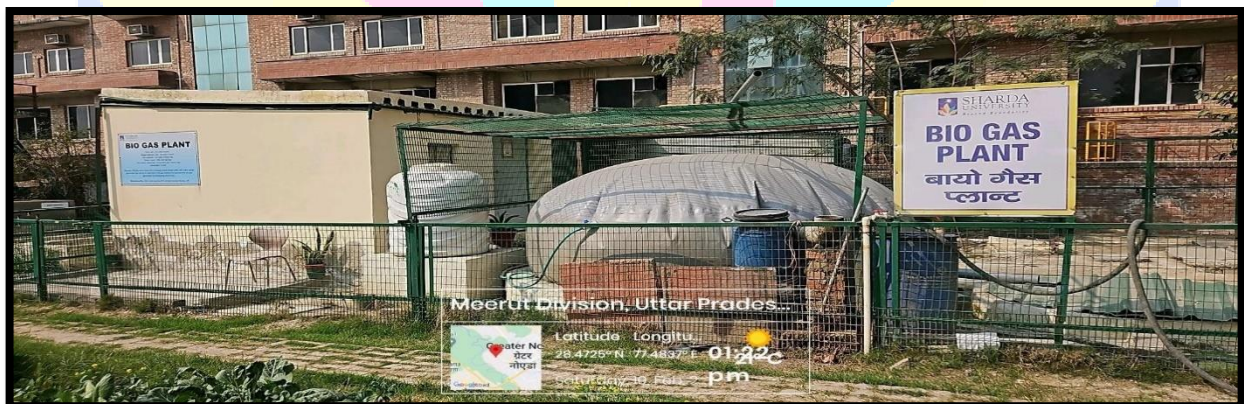
Fig. 9: 5KV Biogas plant of the University
