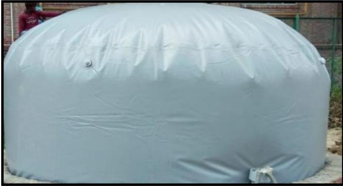
Fig.13: Biogas Plant near Block 7 (Sharda University)
